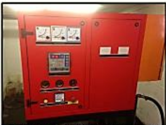
Photo 65 : Scout Camp Sewage Pumping Station : Control panel of Standby power
