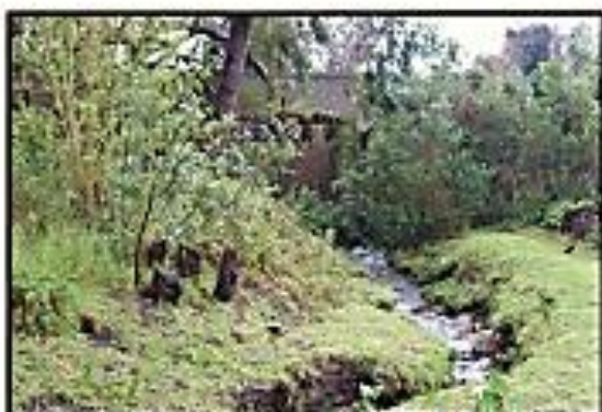
Photo 3 : Stormwater channel west of the Development and at the entrance to De Mond
