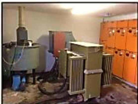
Photo 67 : Mosselriver sewage pumping station : Control panel and transformer
