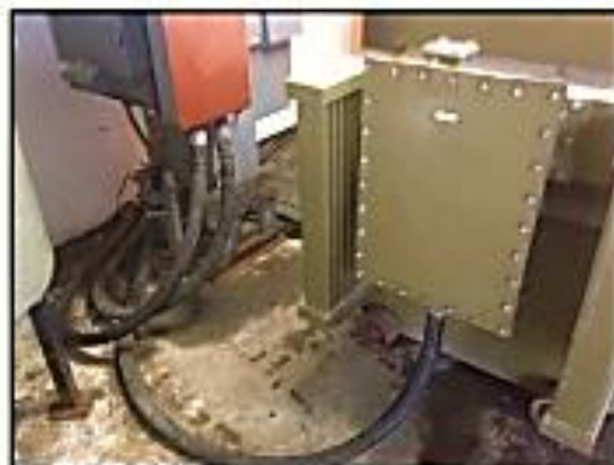
Photo 70 : Mosselriver sewage pumping station : Transformer
