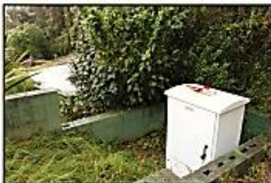
Photo 56 : Control kiosk of existing sewage pumping station at De Mond
