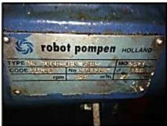
Photo 69 : Mosselriver sewage pumping station : Pumping station
