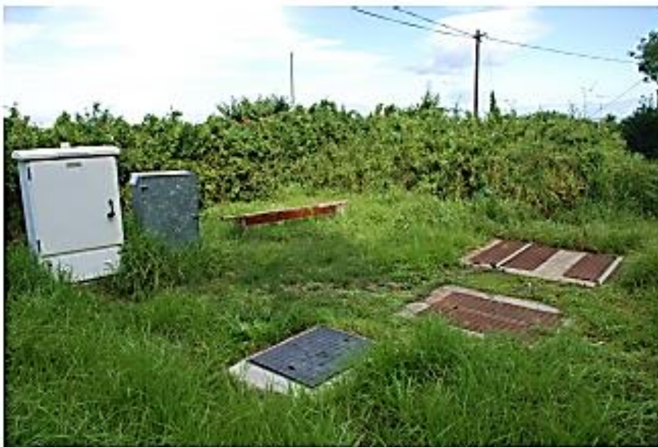
Photo 5: The Caravan Park is serviced by a system of conservancy tanks and pumps which connect with the Municipal sewage reticulation network. This system may need to be upgraded.
