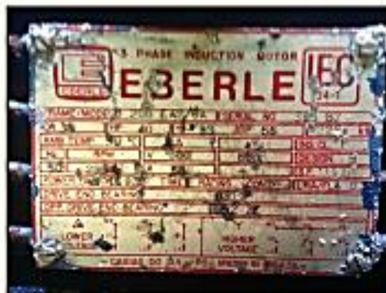
Photo 68 : Mosselriver sewage pumping station : Pump motor information
