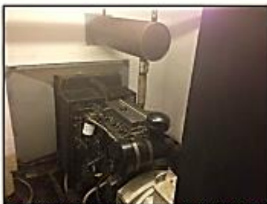
Photo 64 : Scout Camp Sewage Pumping Station : Standby Generator
