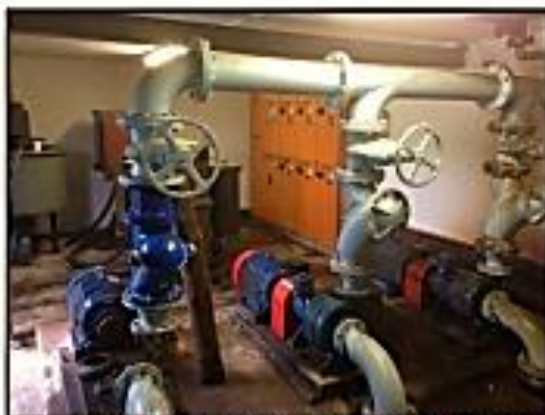
Photo 66 : Moesselriver sewage pumping station : Existing pipework
