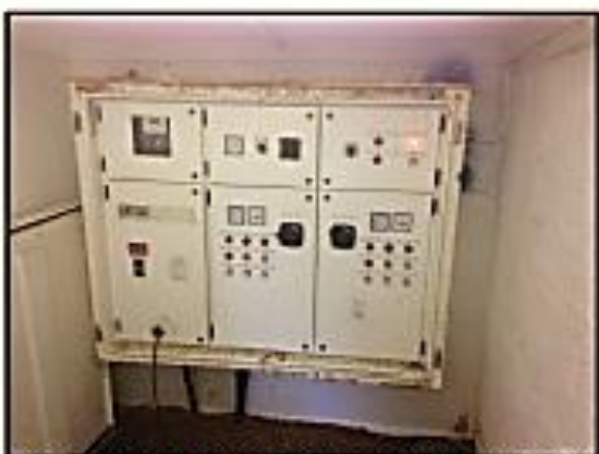
Photo 63 : Scout Camp Sewage Pumping Station : Control panel
