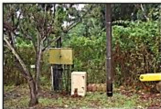
Photo 34 : Electricity kiosk at Klein River Lagoon Park
