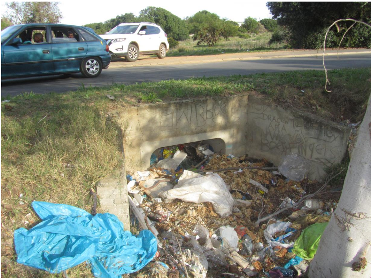
Plate 13. Photograph of the culvert at George Viljoen Street, filled with litter
