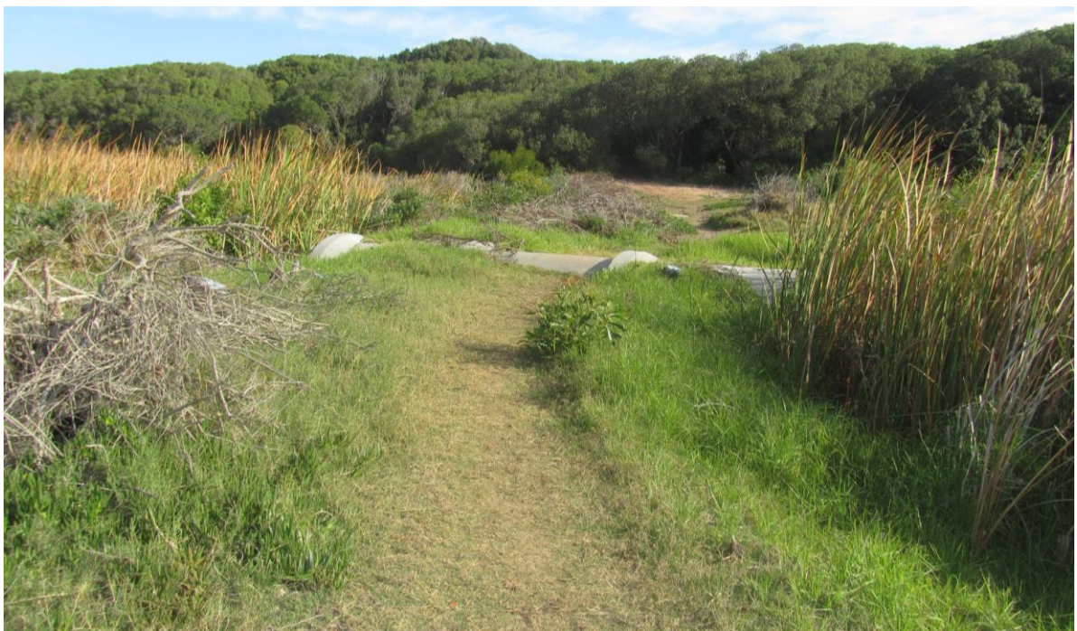
Plate 11. Photograph of the pipe culvert and embankment that separates the core vlei area from the lower section
