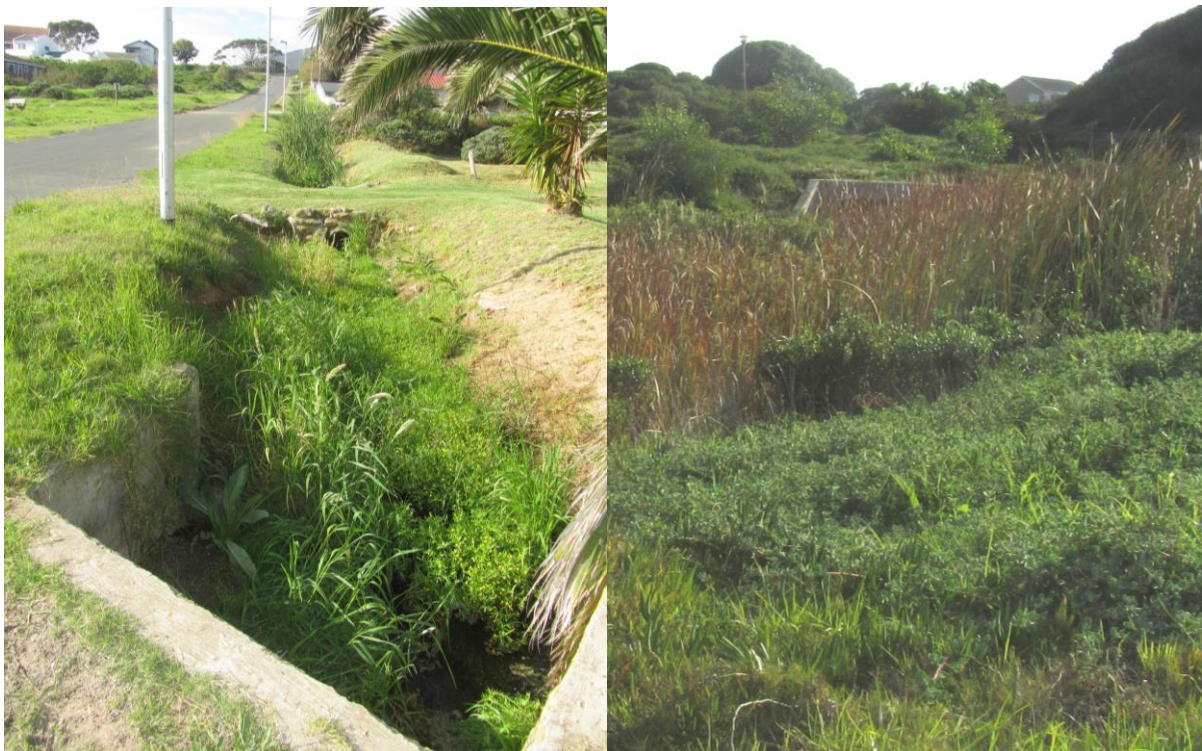
Plate 5. View of the stormwater canal draining into Paddavlei along Vlei Street (left) and the stormwater pipe that installed in the lower Paddavlei
