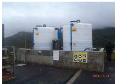
Bunded area for chemical storage tanks
