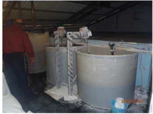
Chemical tanks not banded
