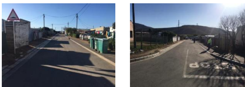
Upgrading of roads Zwelihle, Hermanus
