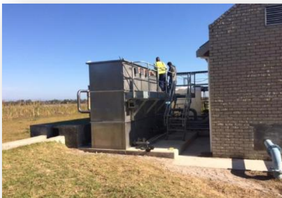
New DAF pre-treatment facility at the Pearly Beach Water Treatment Works (WTW)
