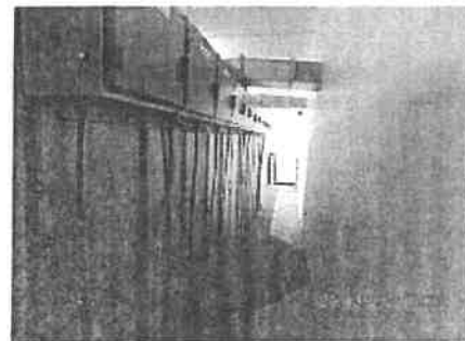
Cable Trenches covered at all areas
