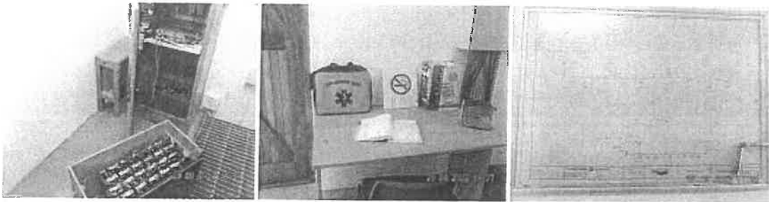
batteries maintained, logbook available and single line available and mounted on the wall.
