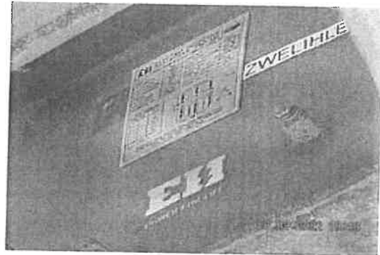
50KVA Electro Inductive transformer.
