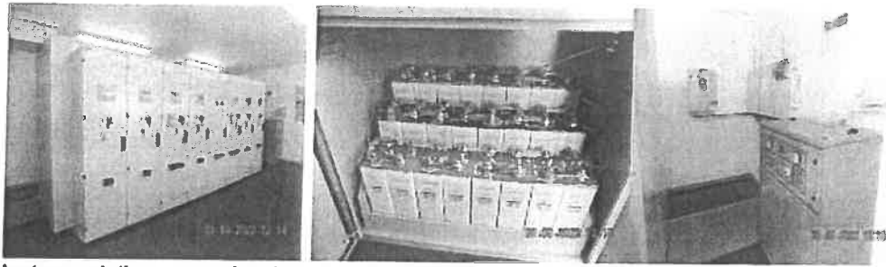
Instrumentation operational and batteries maintained and cable trenches closed at all designated areas.
