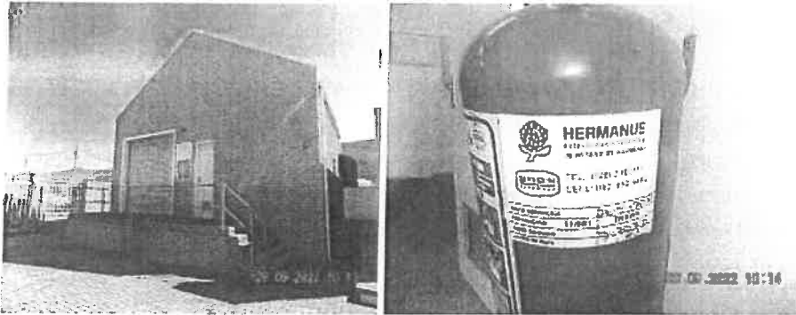
Unauthorised entry controlled by means of a fence, lockable gate and doors. Fire extinguisher service serviced in May 2022.
