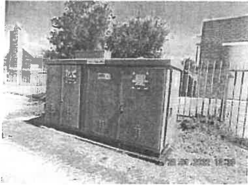
Enclosure was not mounted on a proper plinth.
