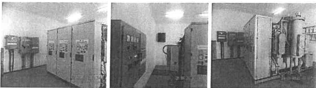
Instrumentation and 66 KV Bus coupler operational and batteries maintained.
