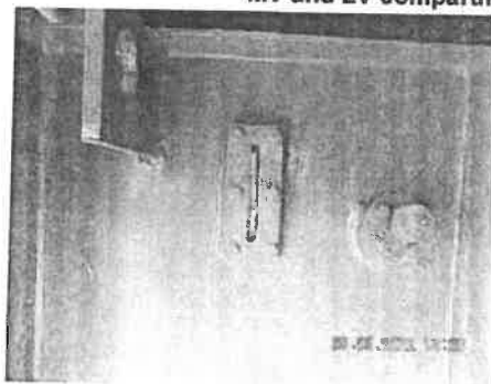
Oil Level on acceptable level.
