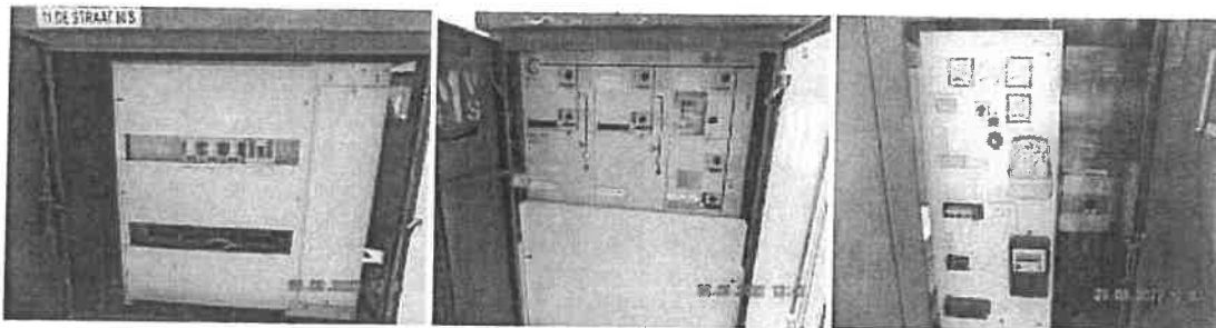
MV and LV compartments were in good condition.
