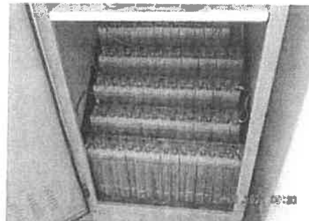
Batteries well maintained and the battery in working condition.
