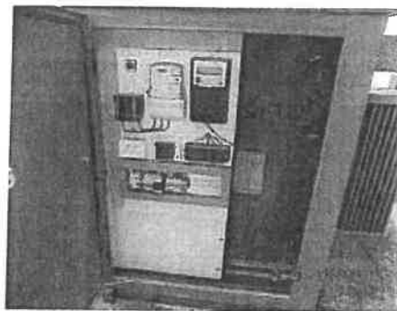
Metering instrumentation functioning.
