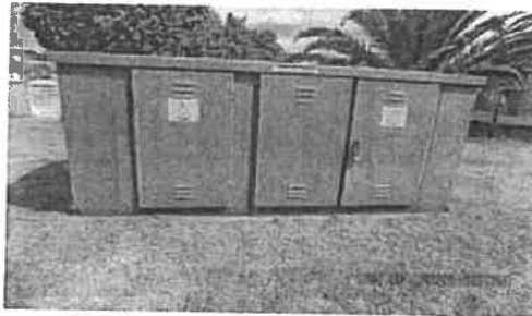
Enclosure secured on plinth.
