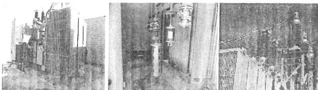
20MVA ABB Transformer manufactured in 2013 was out of service at the time of the Audit.
