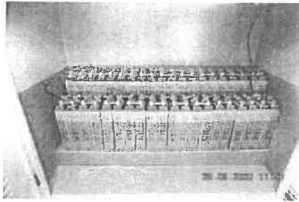
Batteries well maintained.
