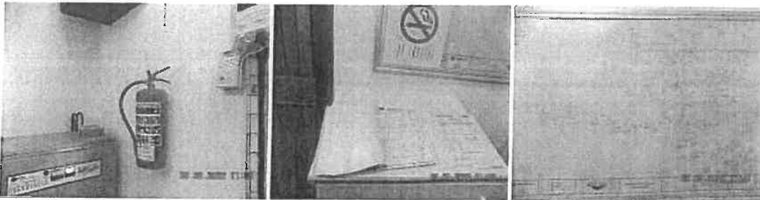
Fire extinguisher serviced, logbook available and single line available and mounted on the wall
