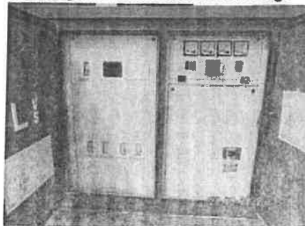
Switchgear in good condition and MV and LV compartments were in good condition
