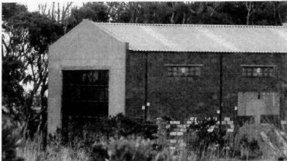
Figure 8: Windows of the proposed tasting room in place. Image taken on 8 May 2021. This doesn't look like the barn for which building permission was requested.
