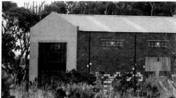
Figure 8: Windows of the proposed tasting room in place. Image taken on 8 May 2021. This doesn't look like the barn for which building permission was requested.
