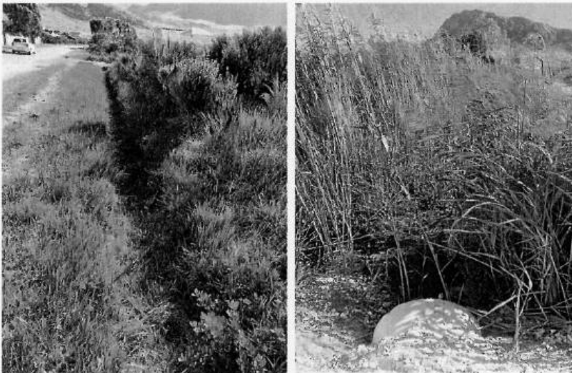
The complete lack of "stormwater" maintenance.
