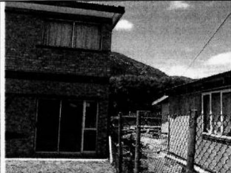
Figure 1: A photo from the rear of the property, of the portion of the building which encroaches on the side building line.
