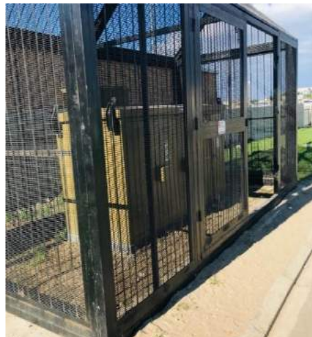
Safe gurading of eletrical transformer (Ward 6)
