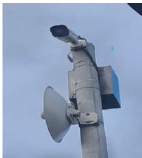
CAMERAS BEING INSTALLED ACROSS THE OVERSTRAND JURISDICTION
