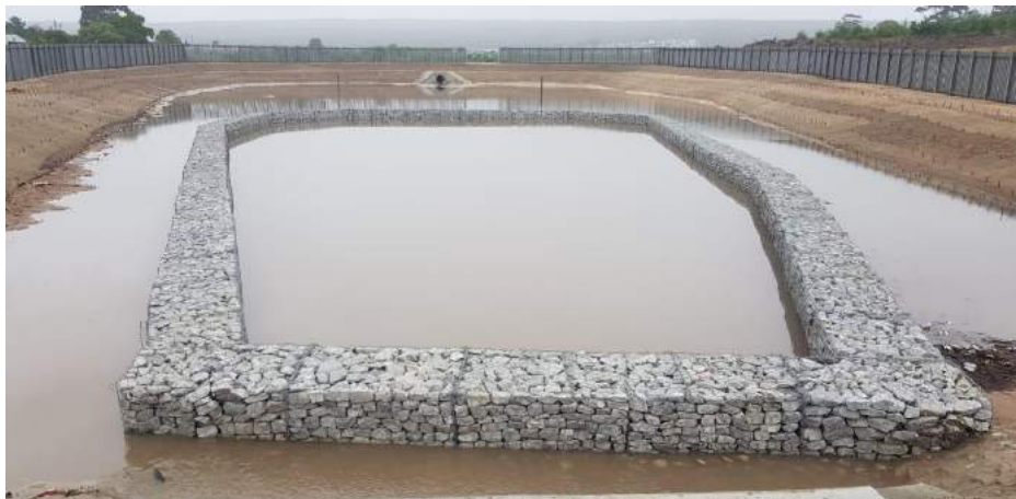
Stanford Housing project Stormwater Pond
