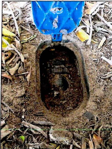
Photo 6: Shared water meter on Portion 2
