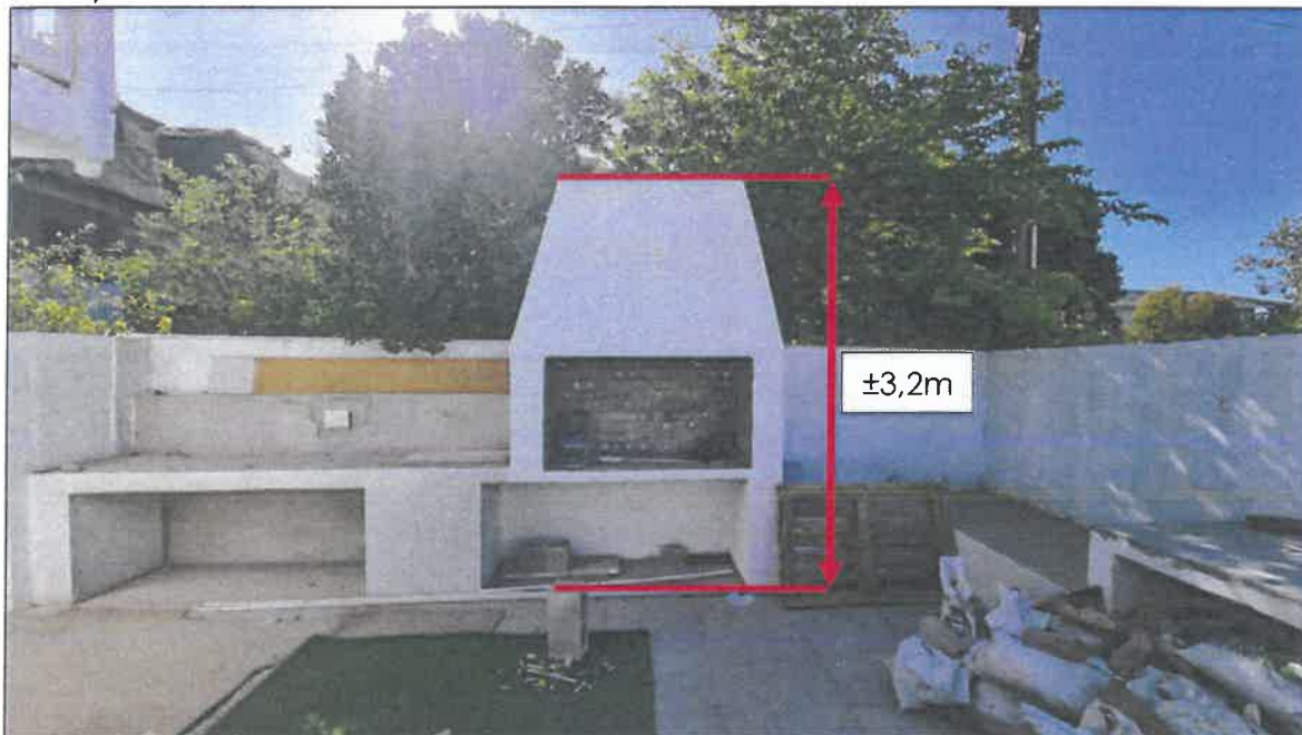
Figure 2: Contravening existing braai
