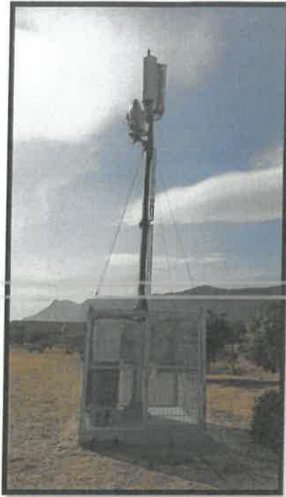
Figure 1 - Existing 9m Transmission Apparatus
