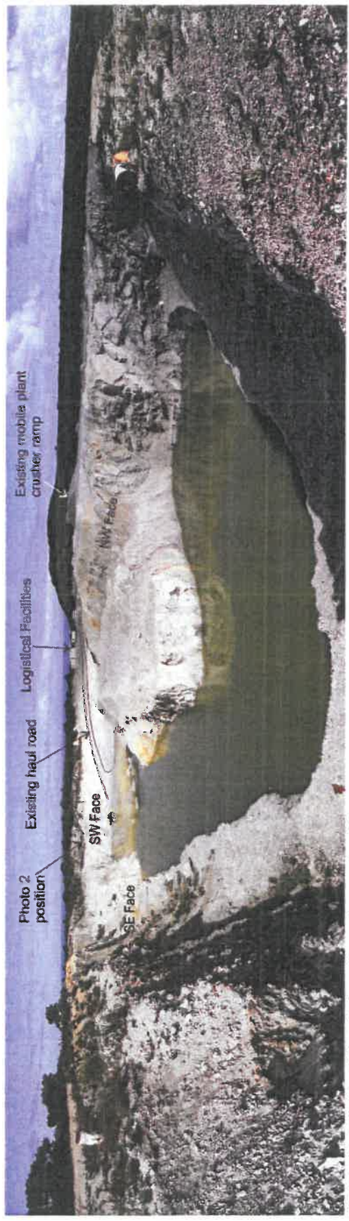
Photo 1: Overall view of the site from the eastern most point of the excavation.
