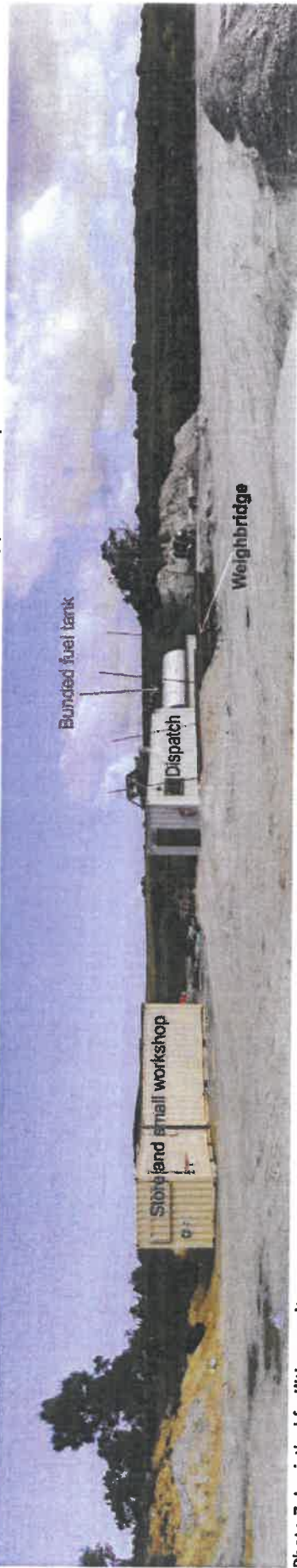
Photo 6: Looking north over the excavation showing the NW/SE slot blasted to achieve optimal advance direction (from safety point of view)
