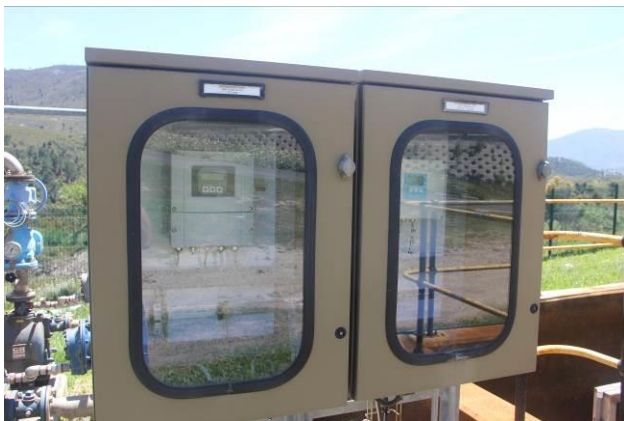
Bulk Mag flow meter for recovery water from Bioplant (Hermanus)
