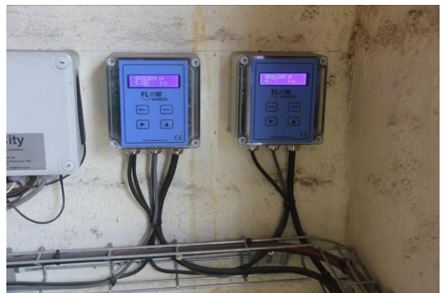
Safmag outlet flow meters for Gansbaai reservoirs, display units
