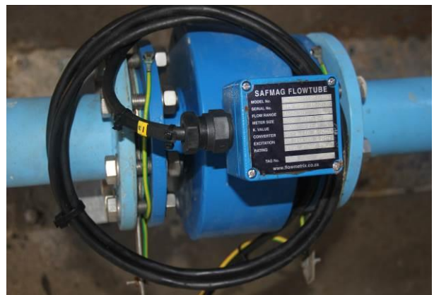
GWP16 Gateway borehole bulk flow meter
