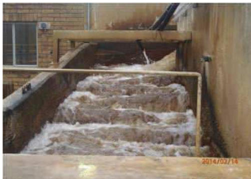
Flocculent dosing at point of high turbulence tanks
