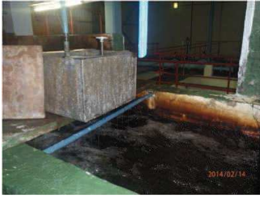
Gravity flow dosing system of flocculent
