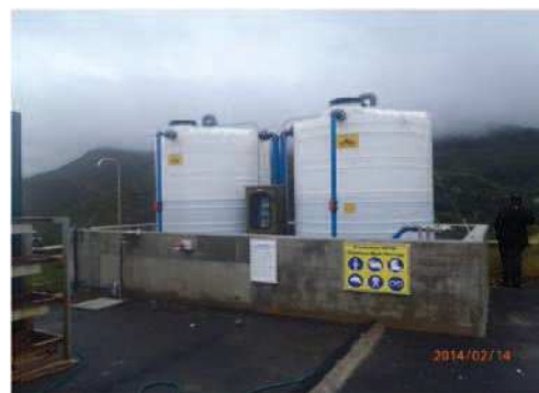
Bunded area for chemical storage tanks
