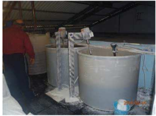
Chemical tanks not banded
