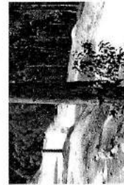
Photo 32: Side drain along the excavation haul road leading to silt trap pond
