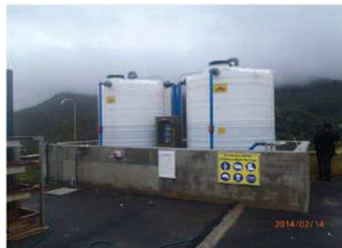
Bunded area for chemical storage tanks
