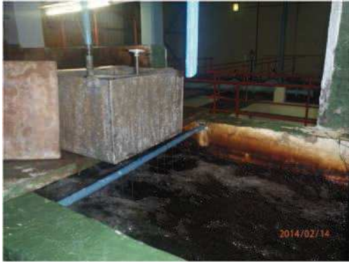
Gravity flow dosing system of flocculent
