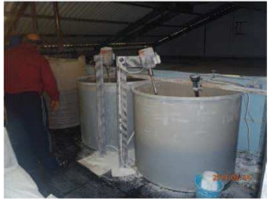
Chemical tanks not bunded
