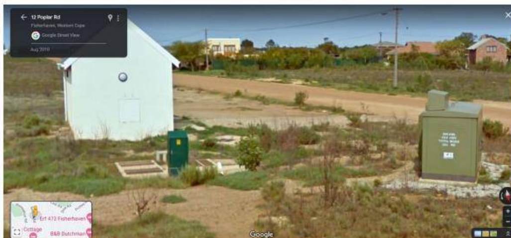
STREET VIEW OF ELEC SUBSTATION
