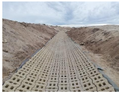
Upgrade of the bulk storm water for Blompark and Beverly Hills housing project, Phase 1 completed
